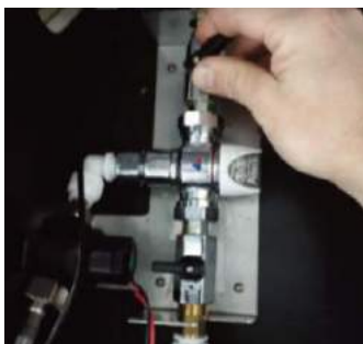
1. Isolate the water supply locally
